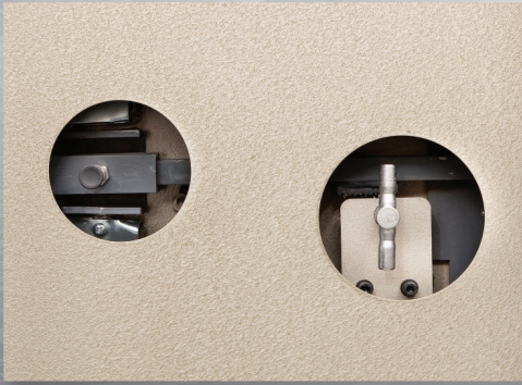
Internal Emergency Door Release
